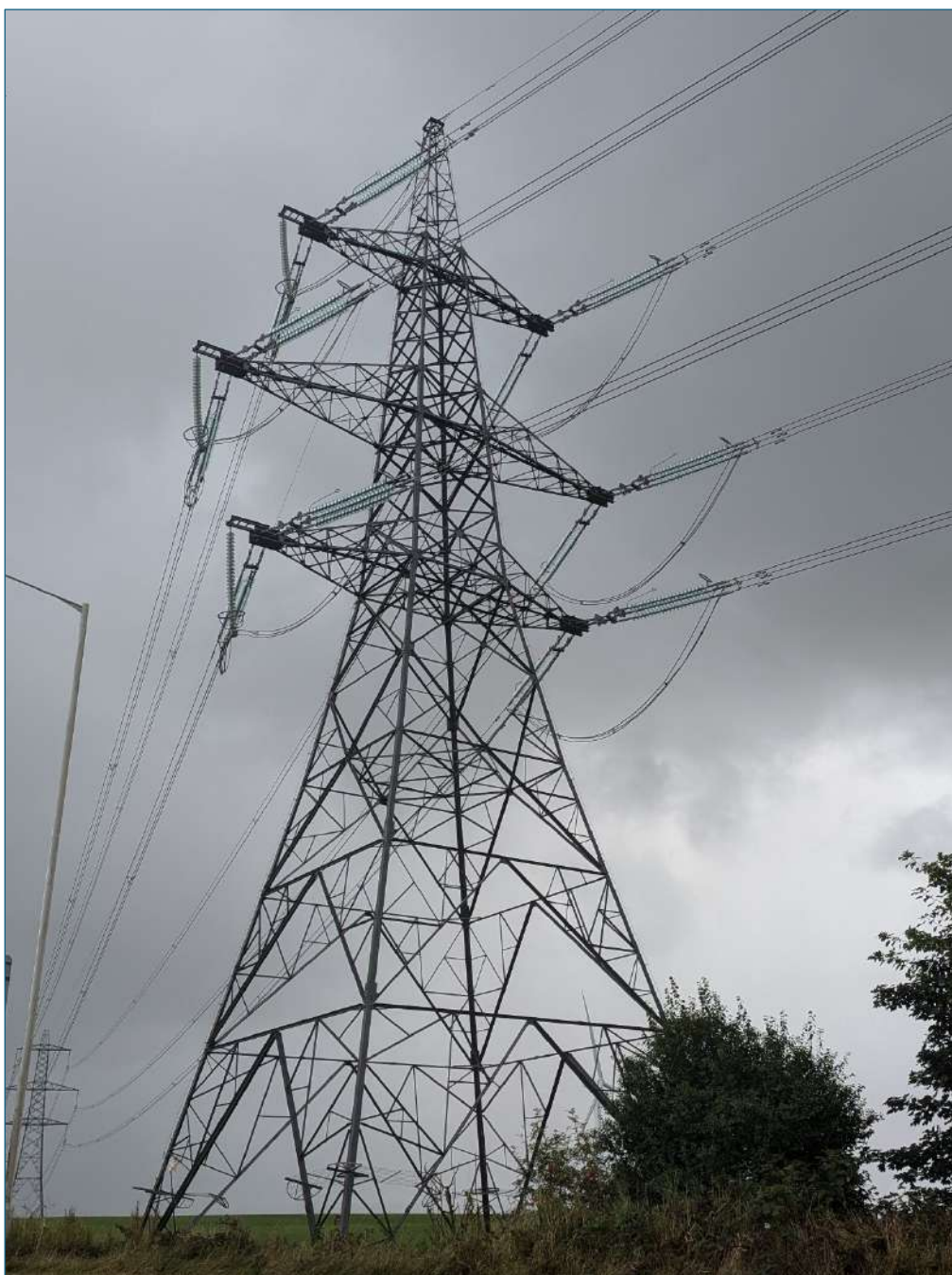
UK National Electricity Distribution Grid, Heysham (400kv), Lancashire, Image credit: Irish Sea Rim
